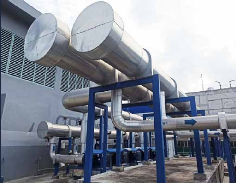
Harco Glodok Chiller Plant ■
